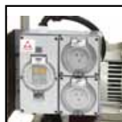
RCD & Weatherproof Outlets
